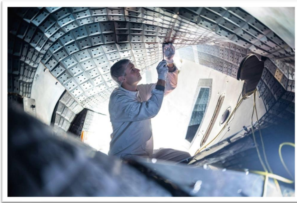
Abbildung 7: Final assembly work in November 2021 on the plasma vessel of Wendelstein 7-X in Greifswald, Germany; Foto: MPI for Plasma Physics / Jan Hosan ↗ https://euro-fusion.org/services/media-library/
